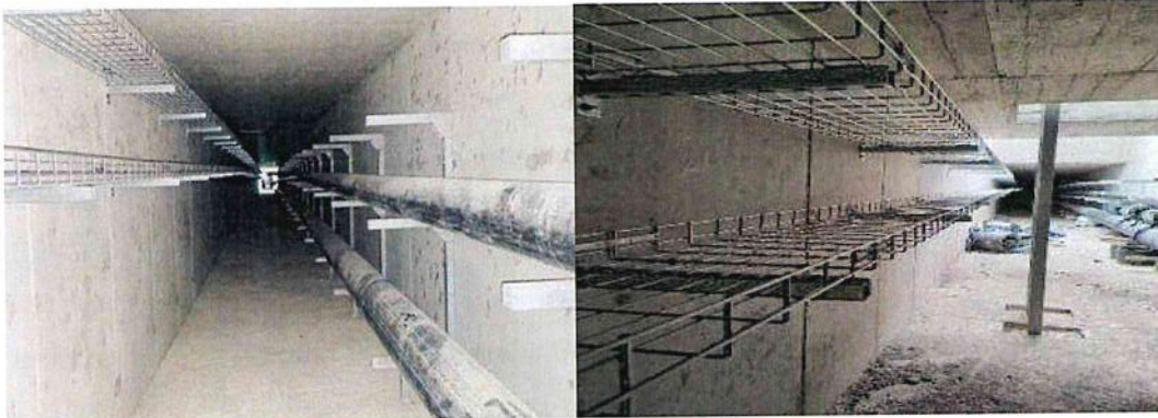
Section of Utility Tunnel in the Technopolis with HDPE pipes and support racks
