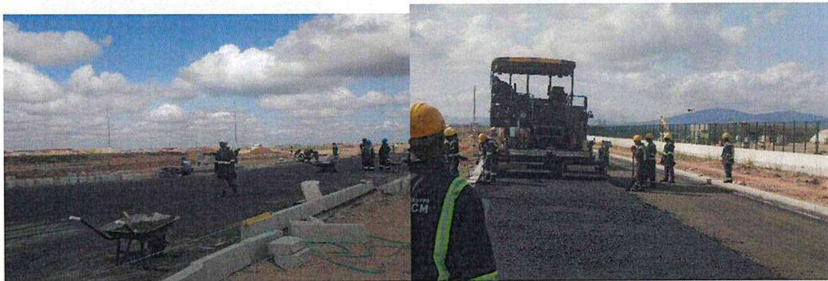
Hunching & installation of road kerbs on Auto Boulevard RHS and Laying of asphalt base course on WRF Road
