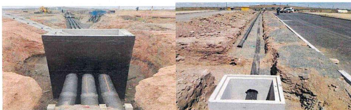
Sand bedding, conduit laying, backfilling, and installation of warning tape from LV-208 to LV-209 on Transit Road.
