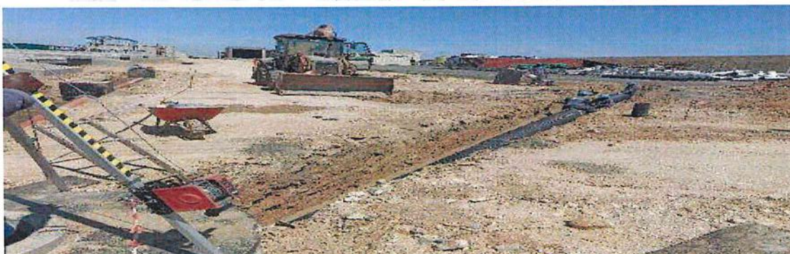
Conduit joining & alignment of stormwater process pipes along the Water Treatment Plant Road
