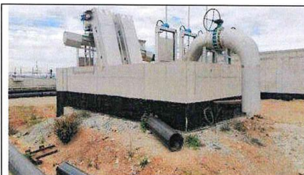
Preliminary Treatment - Mechanical installation
