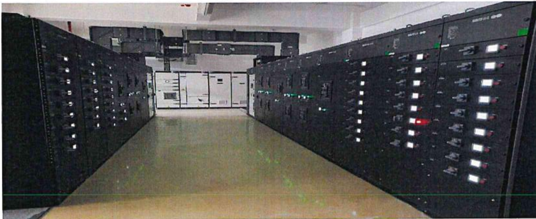
Overview of Electrical room power distribution LV switchgear
