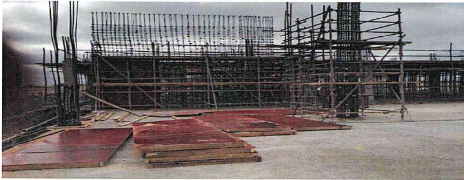
Picture of Police station first floor Ongoing construction works for the police station
