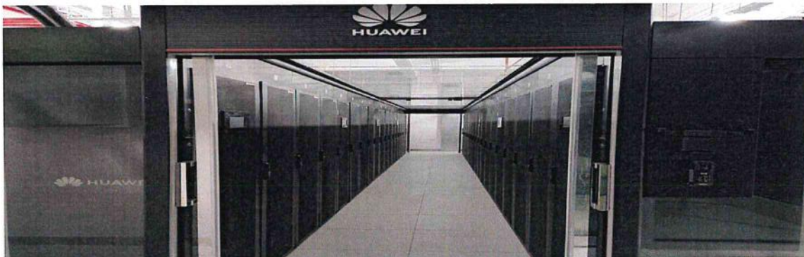
Data centre module 2000 installed
