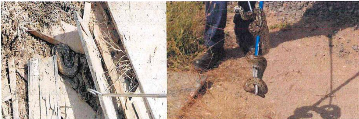
Rescuing of a python from the DS2 Substation and relocation at the Athi-Kapiti ecosystem
