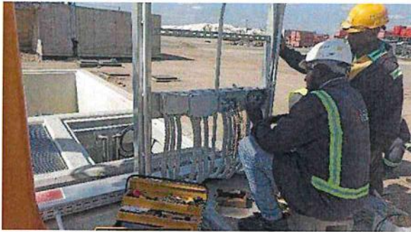
Filter feed pumping station -Pulling of armoured electrical and Trunking of cables
