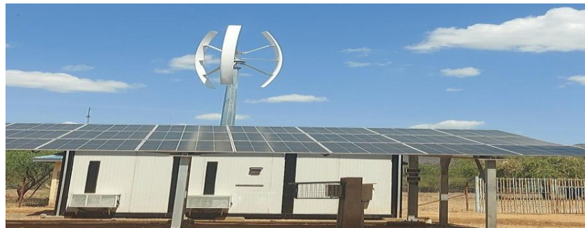
National Optic Fibre Backbone site
