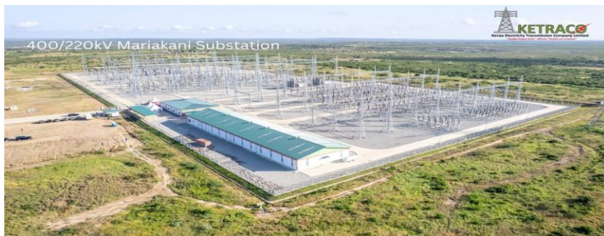
400/220 kV Mariakani Substation, KETRACO, Kilifi County
