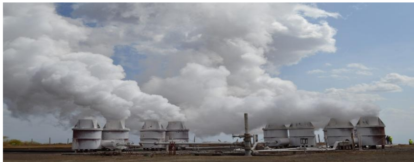
63 MW Olkaria I Rehabilitation, KenGen, Nakuru County
