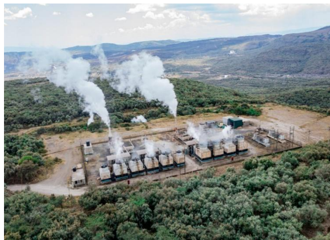
Olkaria Wellhead Generation Plants
